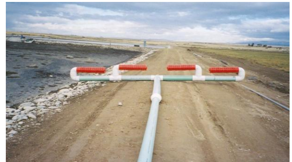
Figure 5. Intake Manifolds (red color perforated pipes), located above the bottom of the lake/pond, for an Absorption Aerator System.
